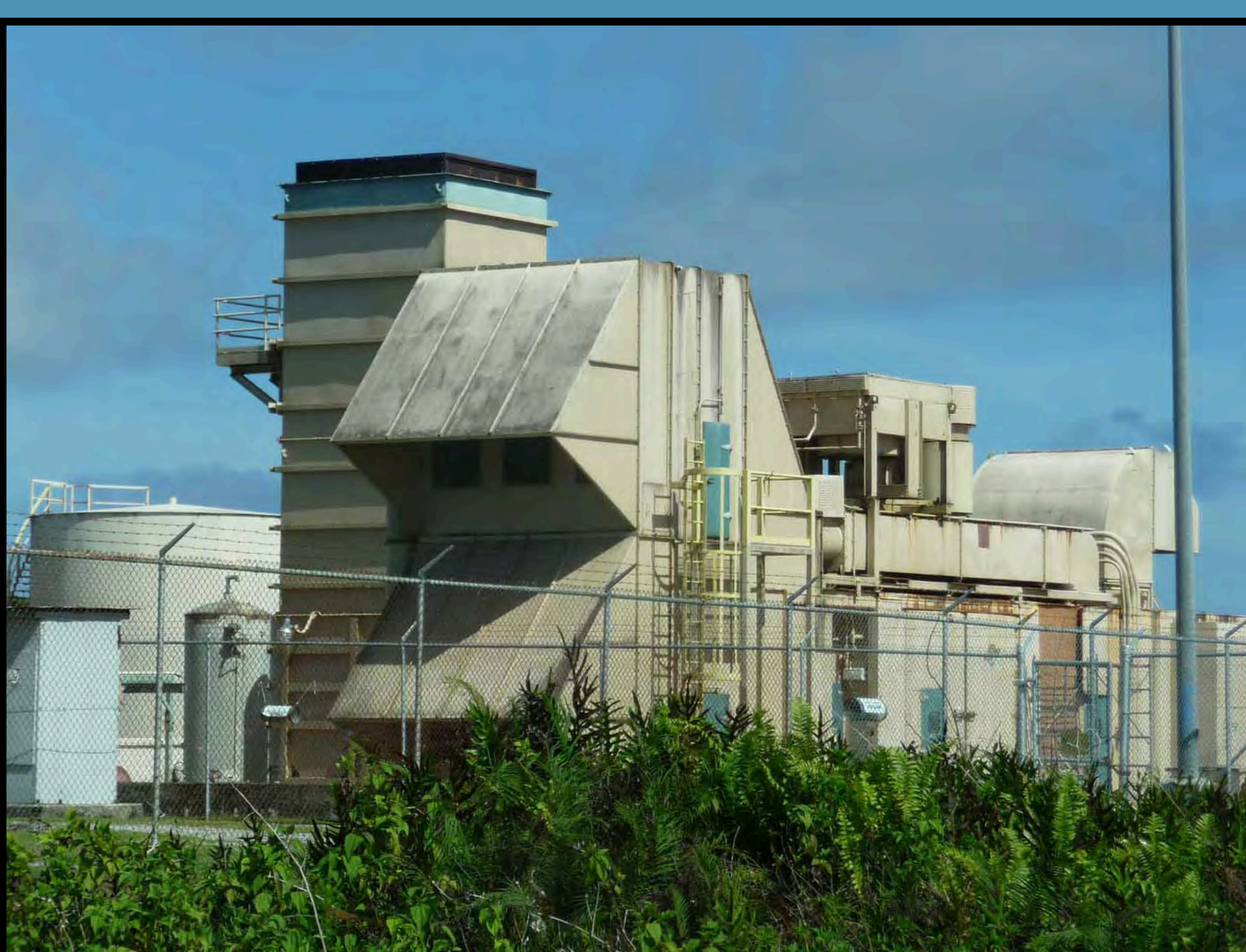
Yigo Power Generation Facility
